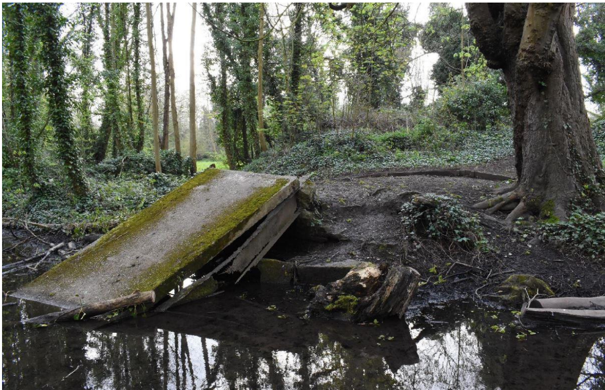
Plate 3. Side view of one of the surviving concrete floors with the metal beam remains underneath (facing East).
