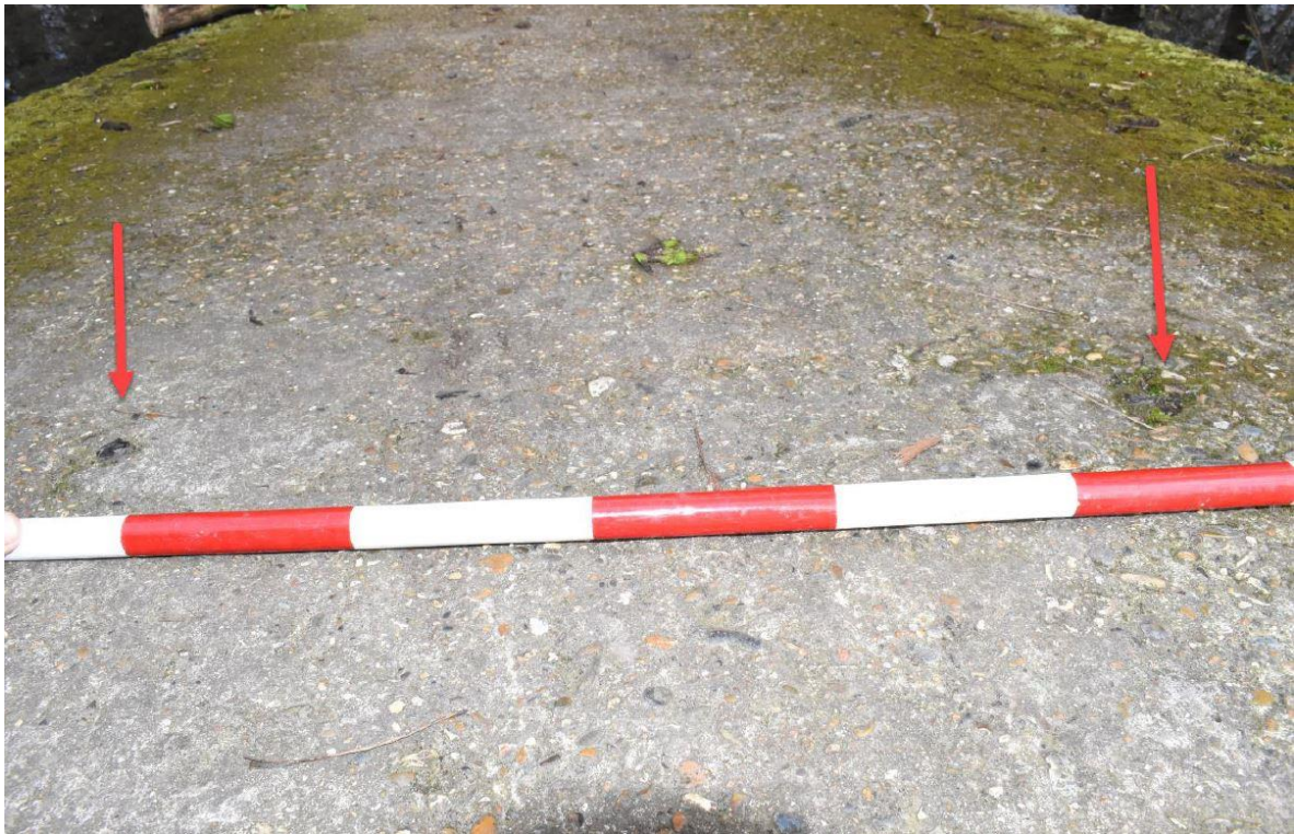
Plate 5. Showing evidence of the metal studs in the concrete floor, Scale 10cm intervals (facing NNW).
